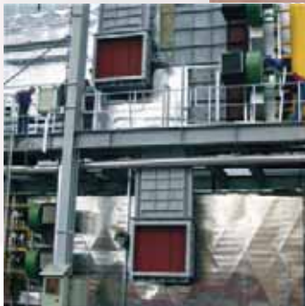
Control valve, sliding gate and gasburner
