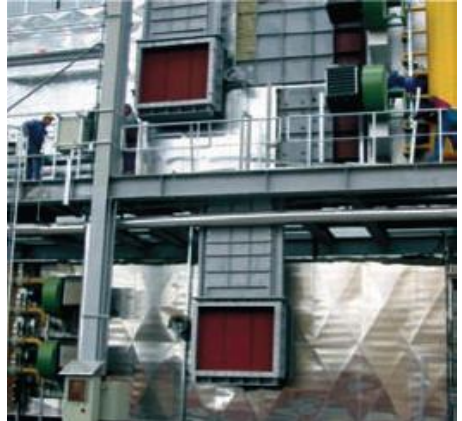
Control valve, sliding gate and gasburner
