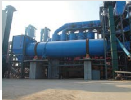
Single stage drum dryer
