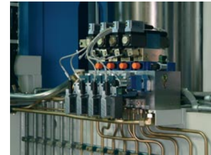
Retrofitting of closed-loop control functions
