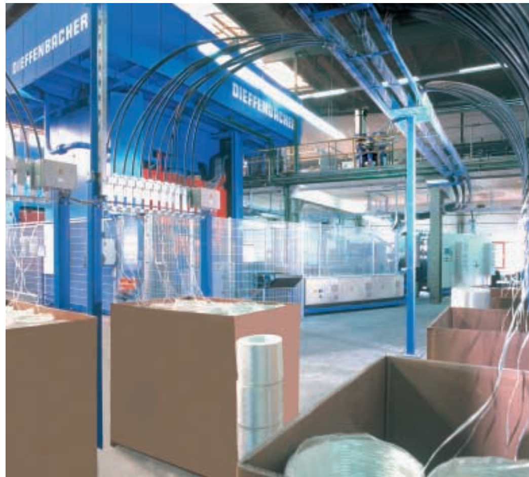
LFT-D line with a 30,000 kN high-speed press equipment with active parallel motion control system
